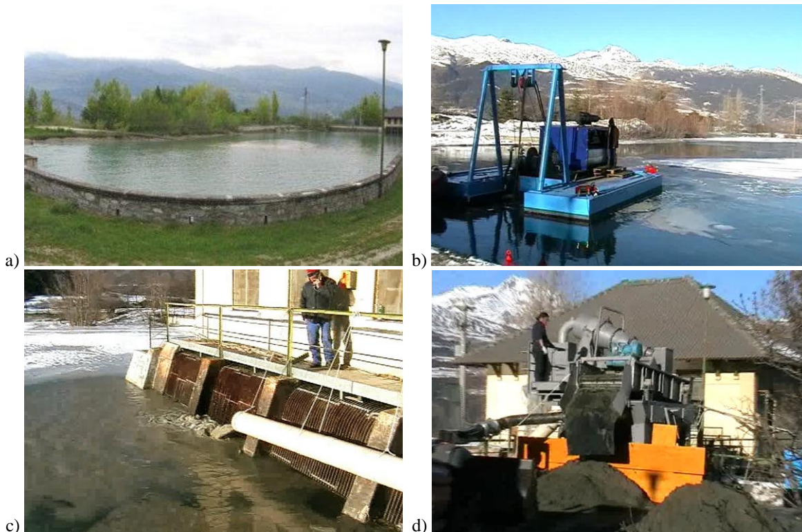
Fig. 5. a) View of the Sorressamont accumulation basin (source: ARPA Valle d'Aosta), b) installation in 2006 of the floating modular unit, c) the introduction of the fine sediments into the water intake and d) the on-shore sediment treatment plant
